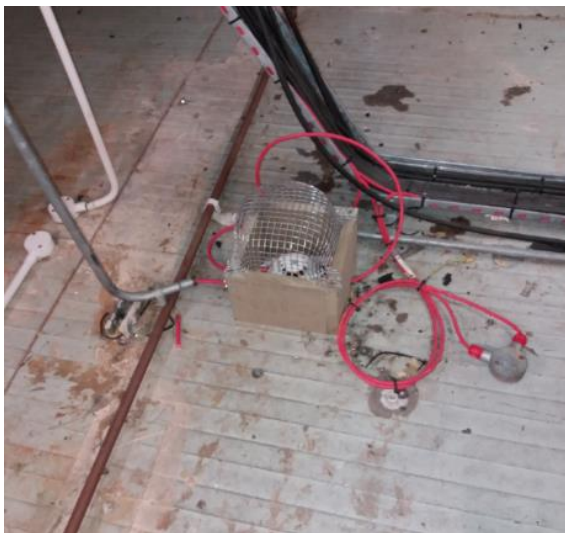
Smoke Detector Head with Protective Box
