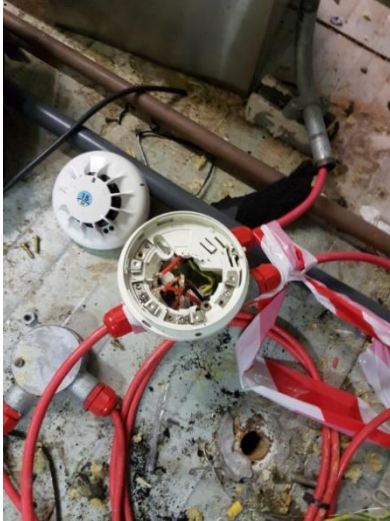
Damaged Smoke Detector Head
