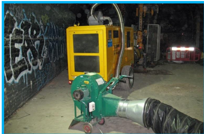
Removal of Exhaust Gases
