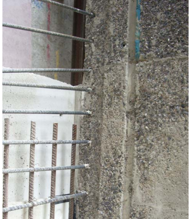
Concrete wall joint after retarder was used and the joint then jet washed
