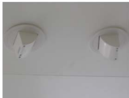
Ceiling Mounted Motion Detectors
